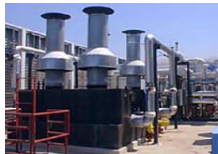
Boiler Plant, Facility A
