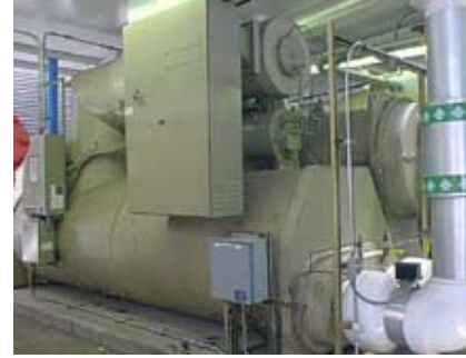
800 Ton Centrifugal Chiller, Facility A
