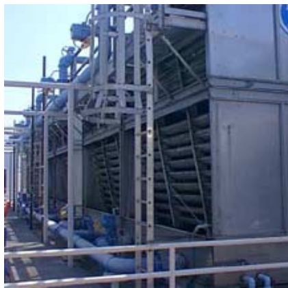
Baltimore Air Coil Cooling Towers
