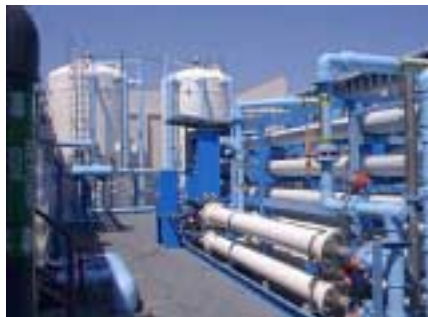
DI Water Plant, Facility A Building 3
