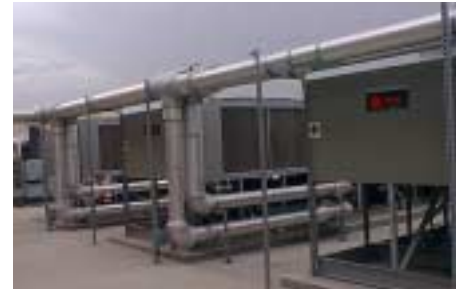
Facility B.1 Air Cooled Chillers
