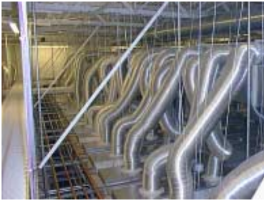
AIT Ducted HEPA System
