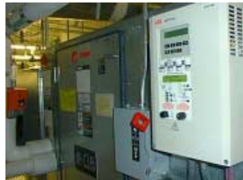
AIT Recirculation Air Handler
