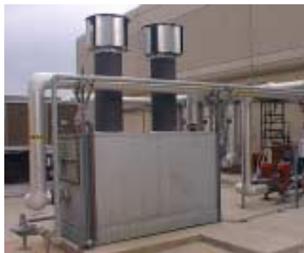
Facility B.1 Boiler
