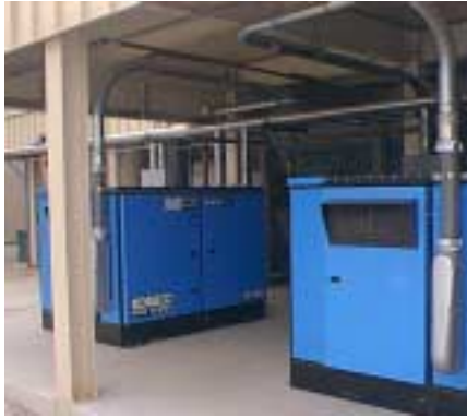
Facility B.1 Air Compressors
