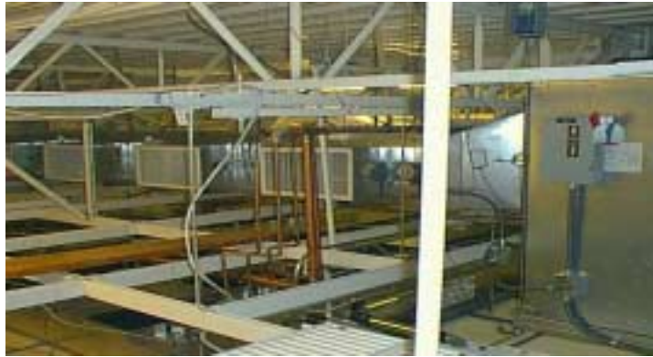
APS/Demo Interstitial Space Recirculation Air Handler and discharge registers above Fan Filter Units
