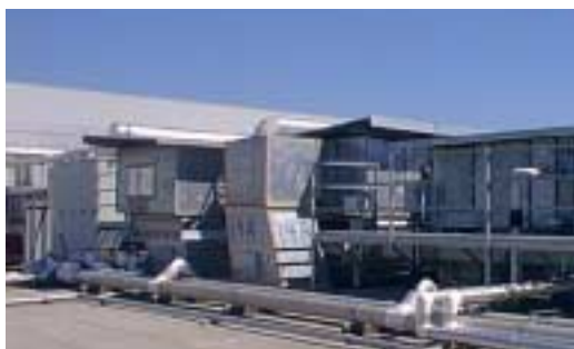
Facility B.2 Recirculation Air Handlers
