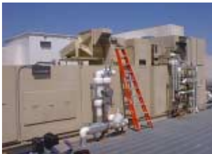
Desiccant Dehumidifier Make Up Air Handler
