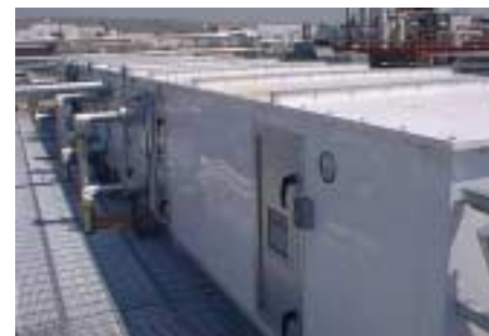
Make Up Air Handler
