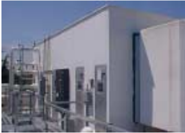
Recirculation Air Handler
