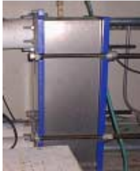
Process Chilled Water Heat Exchanger
