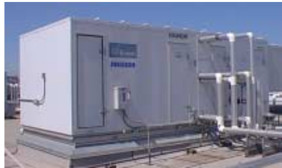
Recirculation Air Handler
